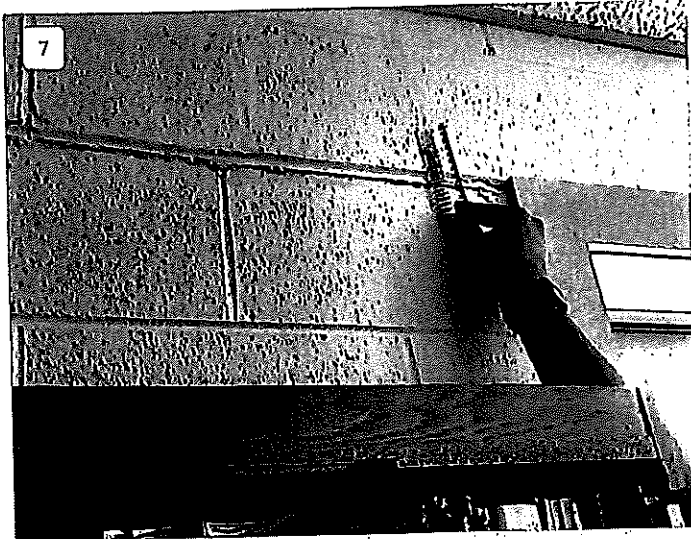
a.7: Width of Cracking (2 of 2)
